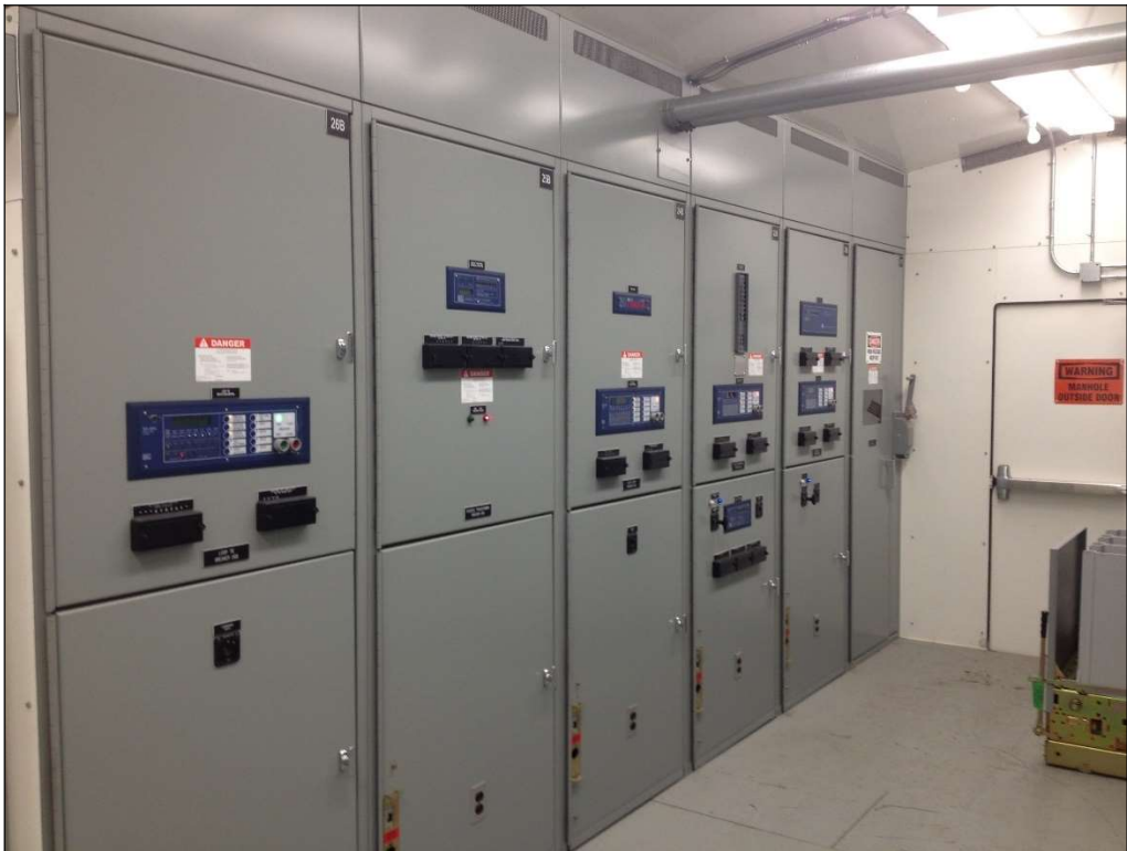
North Street Substation
