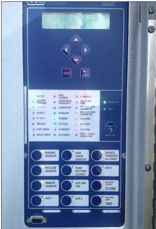
Unit #9 recloser control
