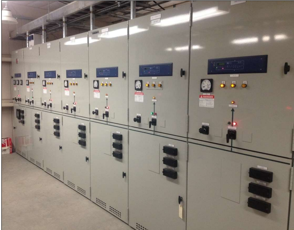
West Substation Switchgear
