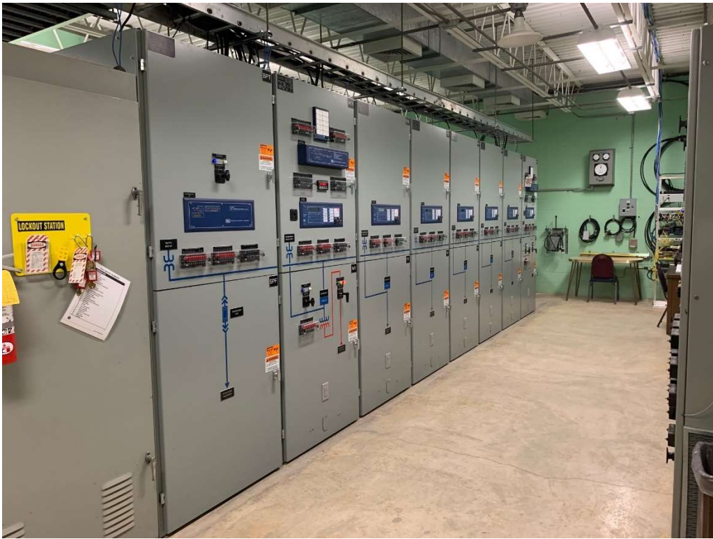
Southeast Substation Switchgear
