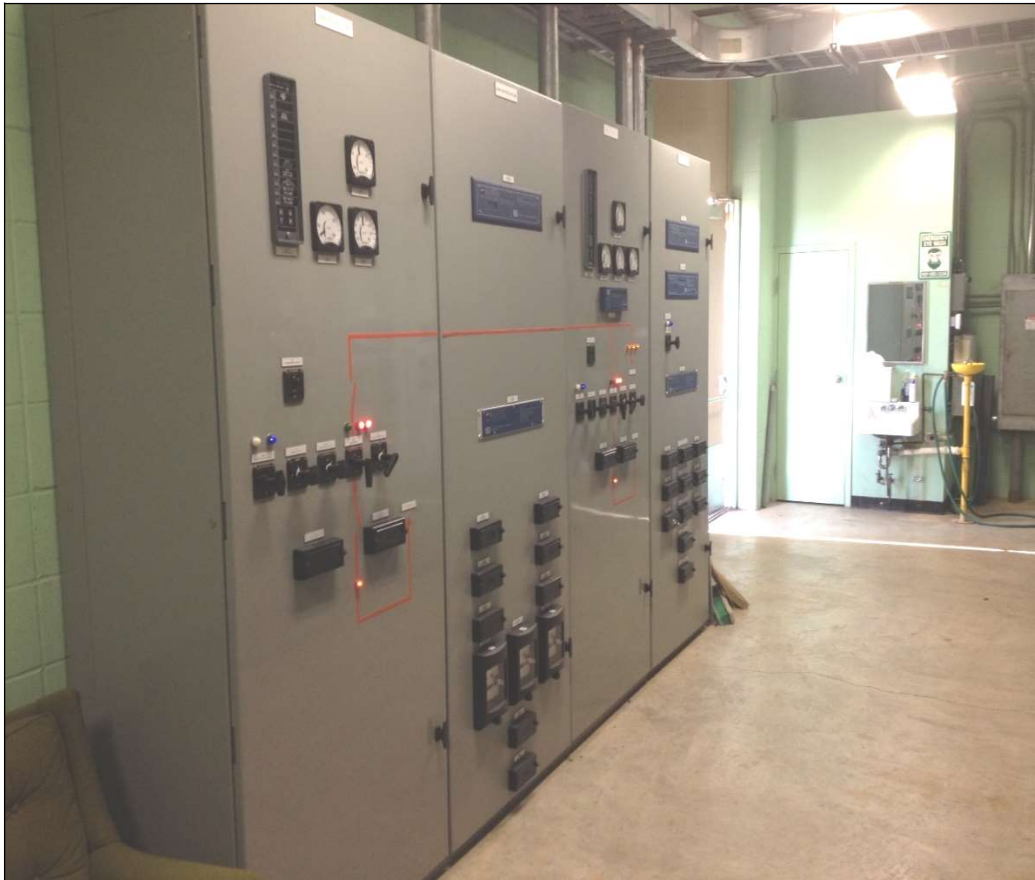
Southeast Substation Transmission Relays
